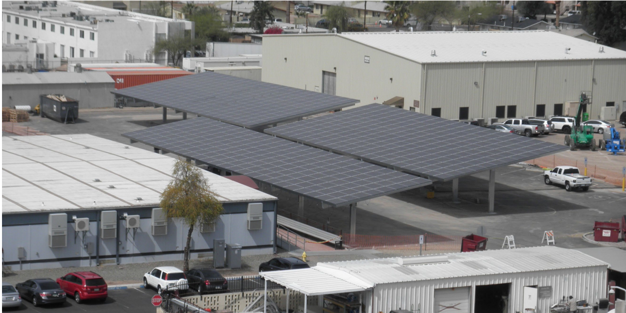
Figure 11. Installed Photovoltaic System at the Phoenix Indian Medical Center
