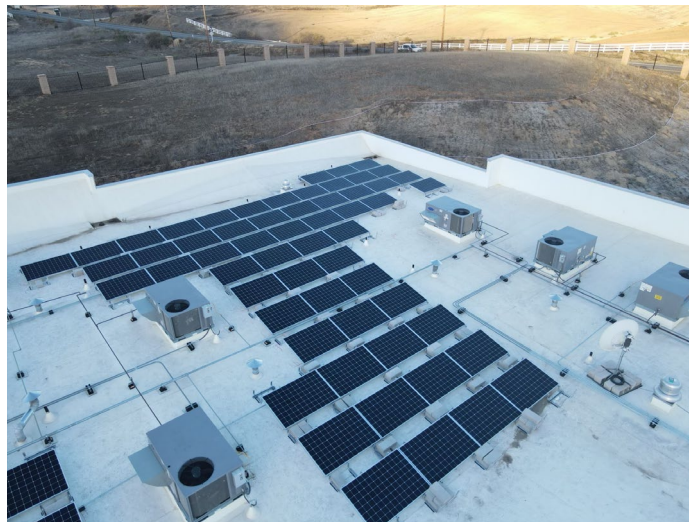
Figure 6. Rooftop PV System at the Pechanga Indian Health Clinic
